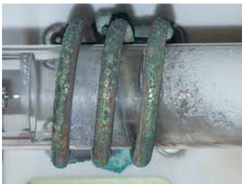
Ready for replacement
